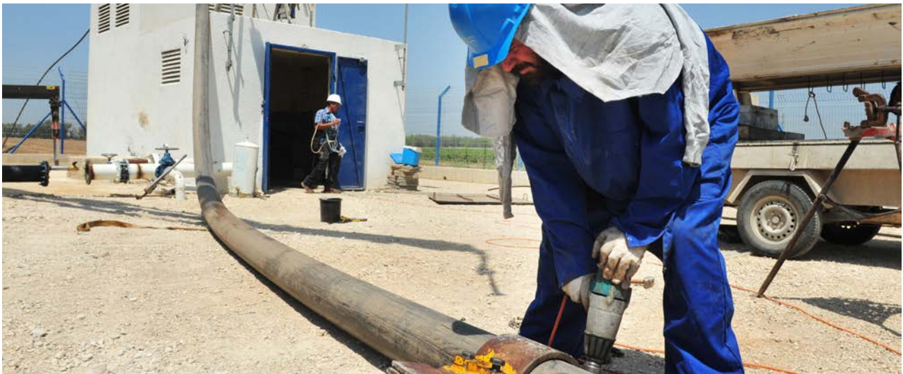
Drilling engineers maintaining water pipe for Mekorot, the national water company, in Ashkelon, Israel. It supplies Israel with 90% of its drinking water and a cross-country water supply. Editorial credit: ChameleonsEye/shutterstock.com
